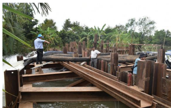
Figure 8. A pumping station for freshwater intake at Tan Phu commune
