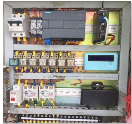
Figure 15. Greenhouse system control cabinet
